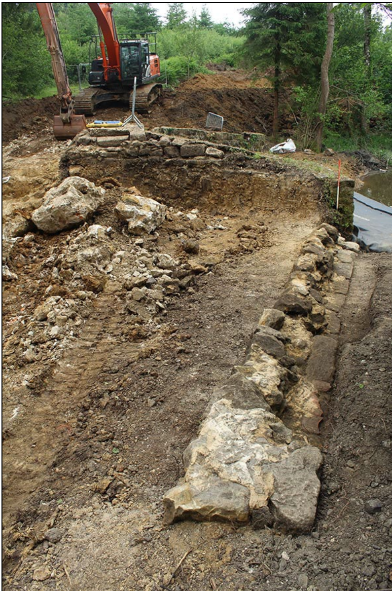
Figure 24 The northern of the western wing walls to the spillway, looking south
