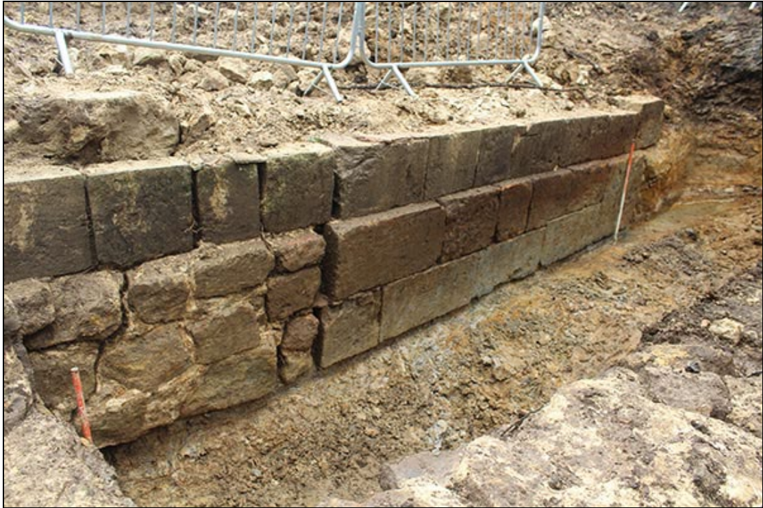
Figure 12 The lowest courses of the north end of the main east wall of the spillway, showing the undressed section of wall in the foreground
