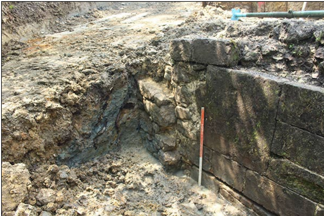
Figure 17 The remains of the earlier wall adjacent to the southern wing wall on the eastern side of the spillway, looking south-west
