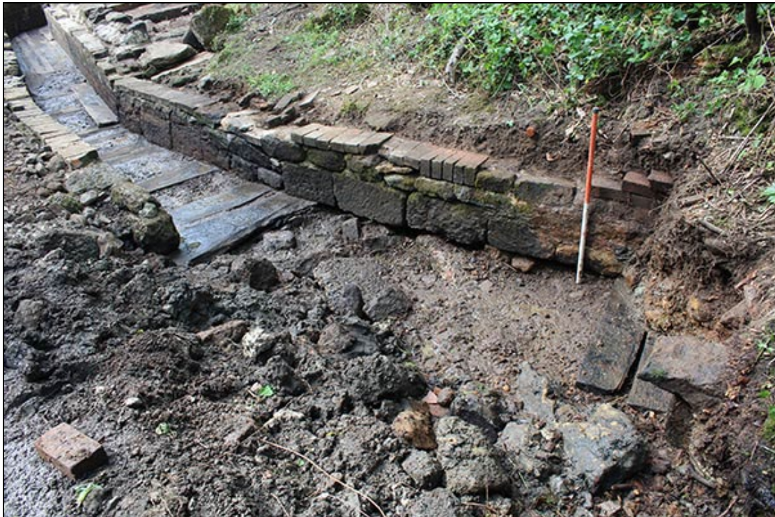
Figure 8 The east end of the tail race, to the right it continues into the slumped bank.
