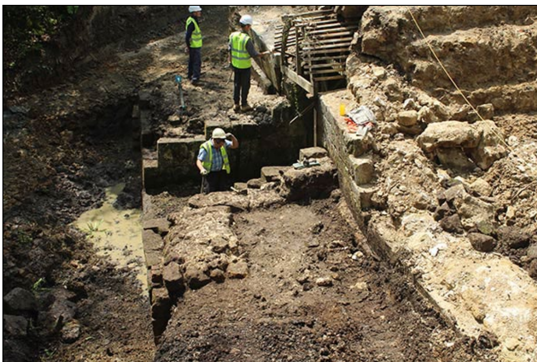
Figure 14 The top of the north wing wall on the eastern side of the spillway, looking south
