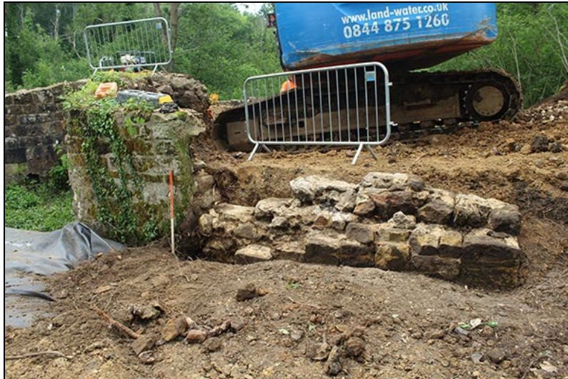
Figure 23 The southern of the western wing walls to the spillway, looking east
